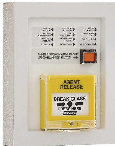
Figure 3: Local Control Station
