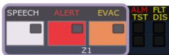
Figure 5-4 Emergency zone with controls highlighted.
